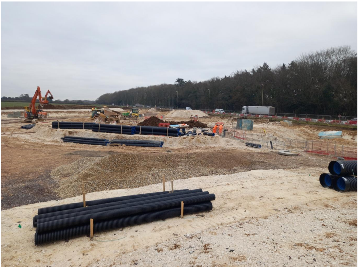
Construction of the Broadway Roundabout to connect to the west of the A32.
